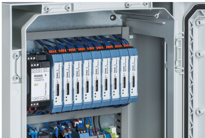
Installation in a control cabinet
